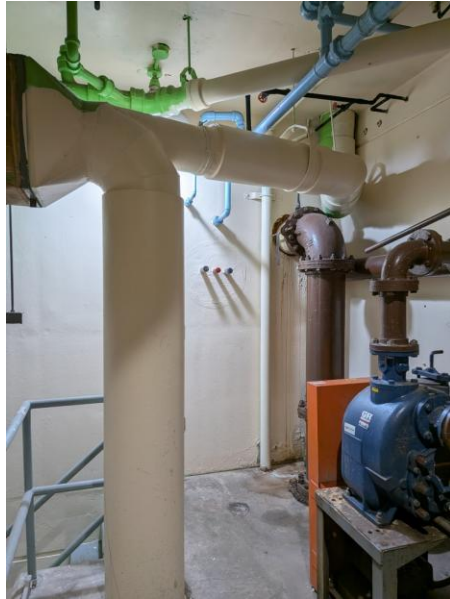
Transite piping on 1 st basement level.
