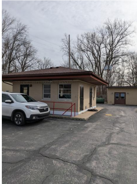
Headworks Building – glaze on windows and doors contains asbestos.
